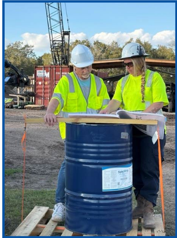
Toho employees review blueprints for expansion of South Bermuda Water Reclamation Facility
